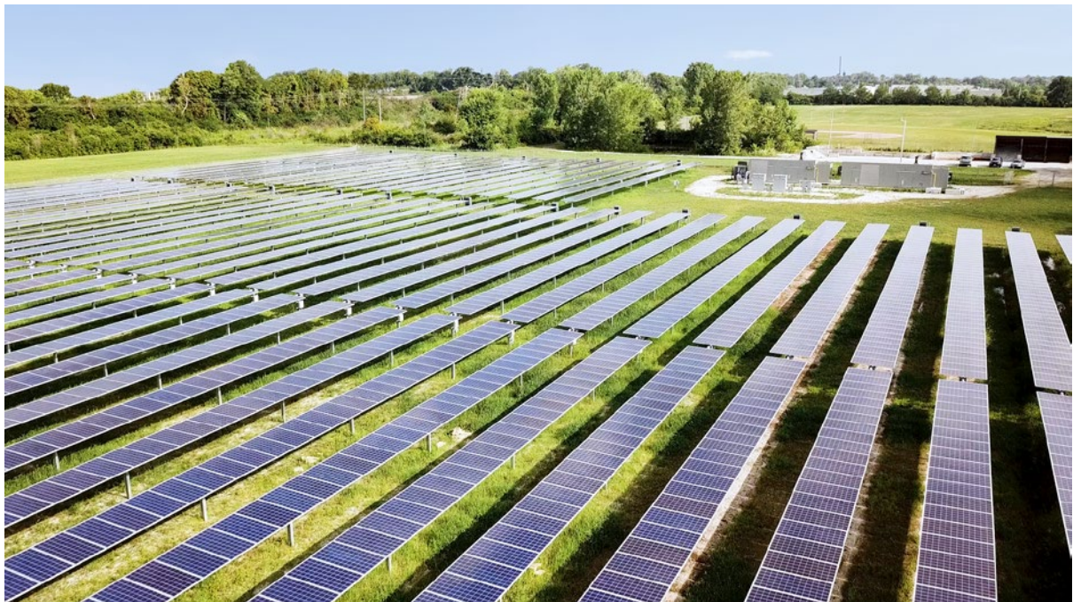
▲ The 2 MW solar, 1.5 MW gas hybrid microgrid system at Ben Davis High School in Indianapolis, Indiana, USA. DEIF controllers manage a peak shaving operation with the intention to save 70% off the school's electricity bill.
