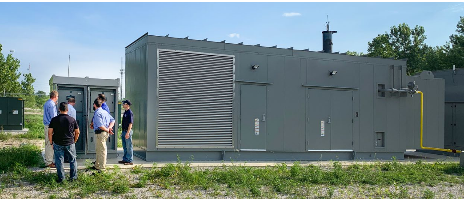
▲ The project team inspects the cabinets and switchgear for the DEIF ASC-4 solar hybrid controllers – adjacent to the gas gensets and main system controls.
